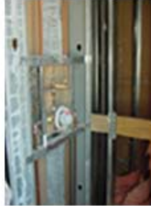
This shower rough-in includes the on-off-volume control valve, and a diverter valve to alternate between the wall-mounted showerhead and the hand-held shower spray
