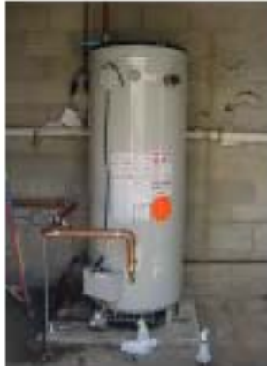
Lochinvar LP-gas water heater of 250-gallon capacity
