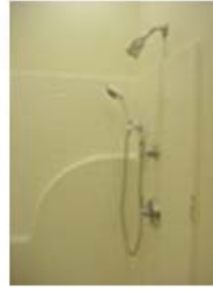
Finished shower is handi- cap-accessible and has a hand-held spray as well as a regular showerhead
